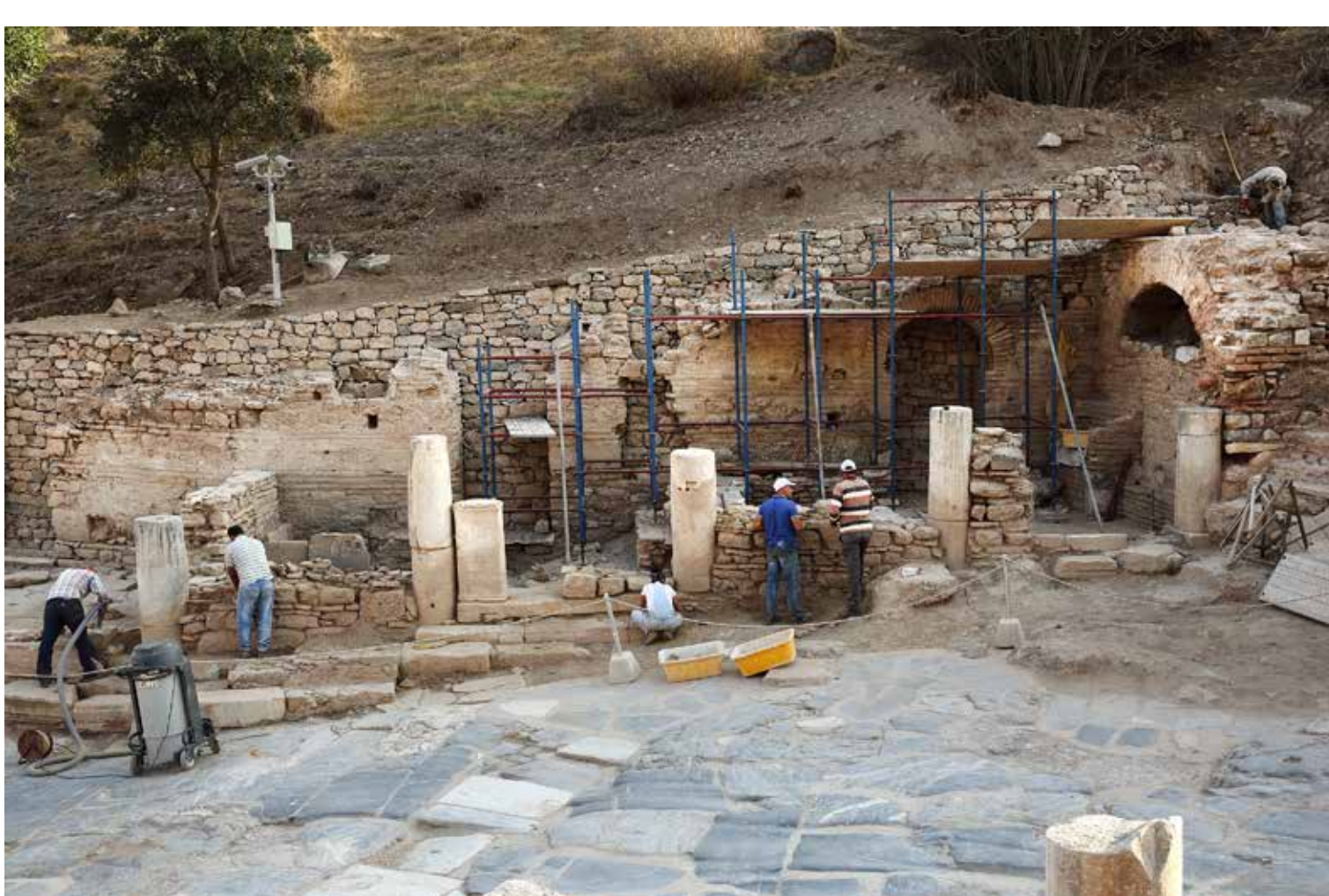
Fig. 6 – Team of workers erecting dry stone walls on Curetes street. (© N. Gail ÖAI/ÖAW)
